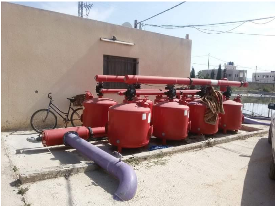
Figure 8. Gravel filters in Jenin's WWTP (Field visit, 2020)
