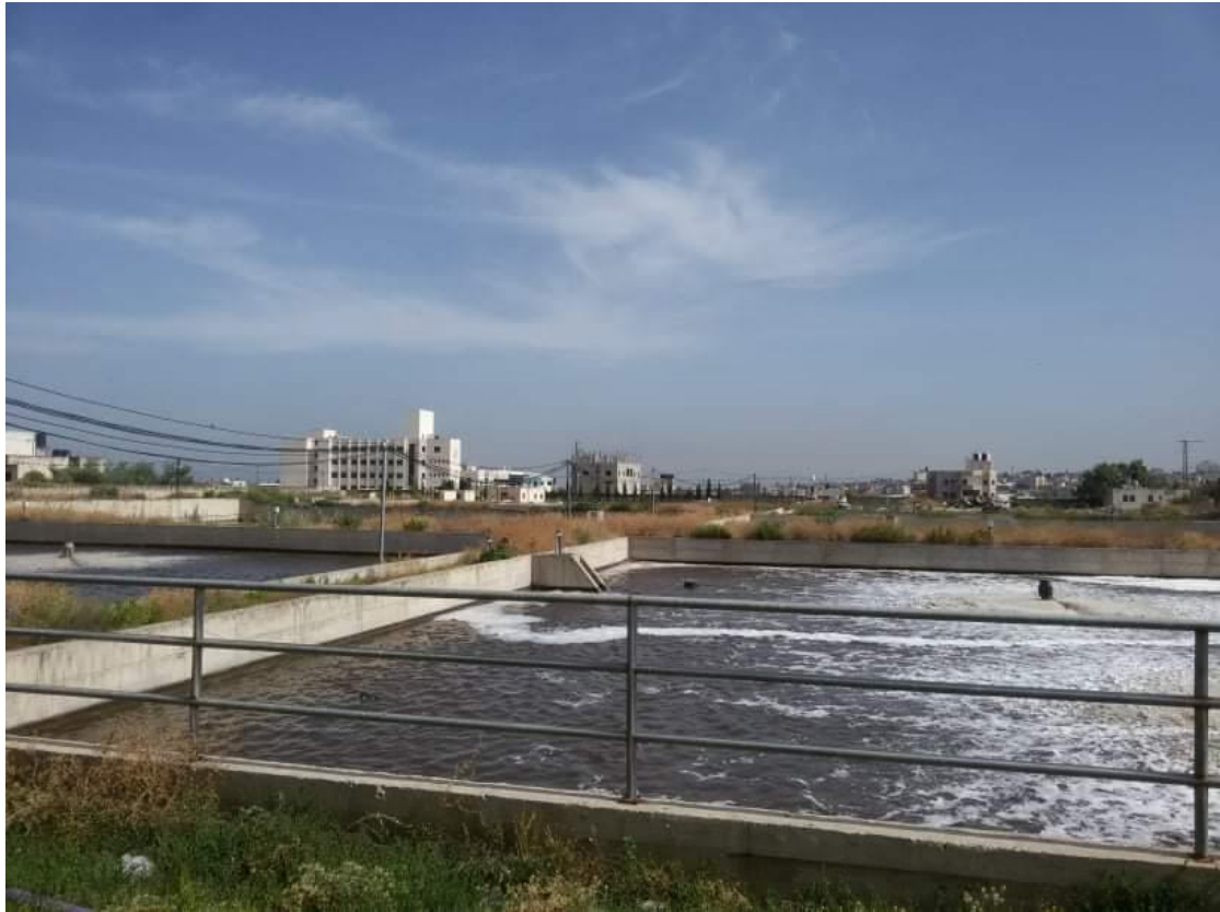
Figure 7. The aerobic biological treatment section in Jenin's WWTP (Field visit, 2020)
